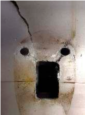
The spreader bar hole in the mast showing corrosion, fatigue cracking and final failure
