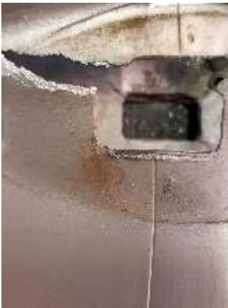
The spreader bar hole showing the area of failure coming from the corner
